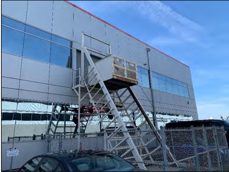
Figure 5.3-11 Building 4, Utility Lift to Second Floor at the Northeast Façade View toward the northwest.
