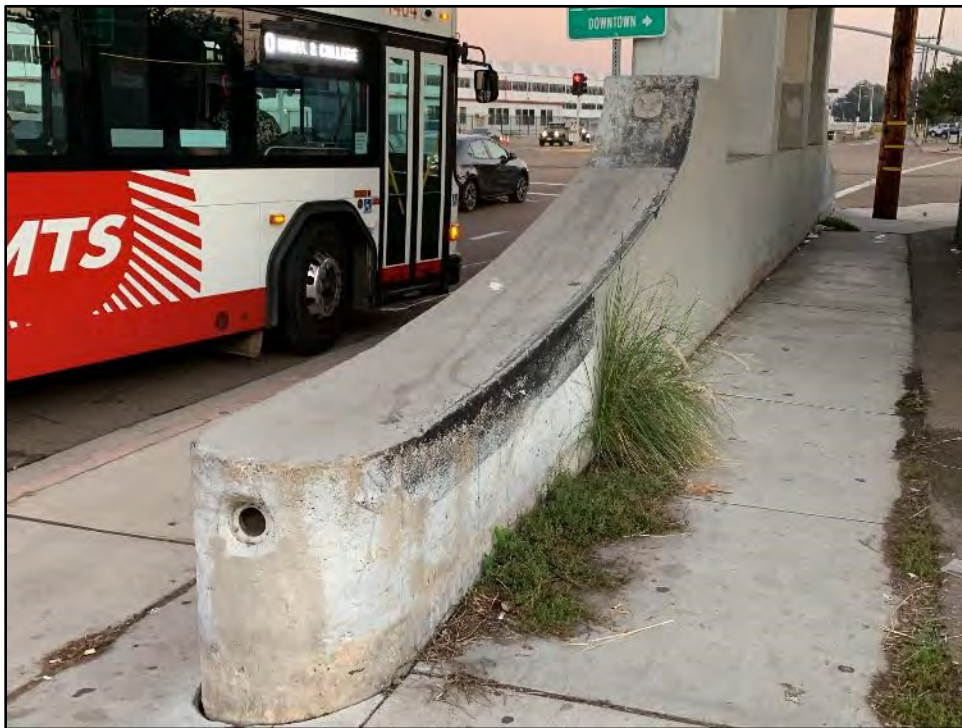
Figure 5.13-8 Detail of the Side of a Support on the Southwest Side of Pacific Highway View toward the southeast.
