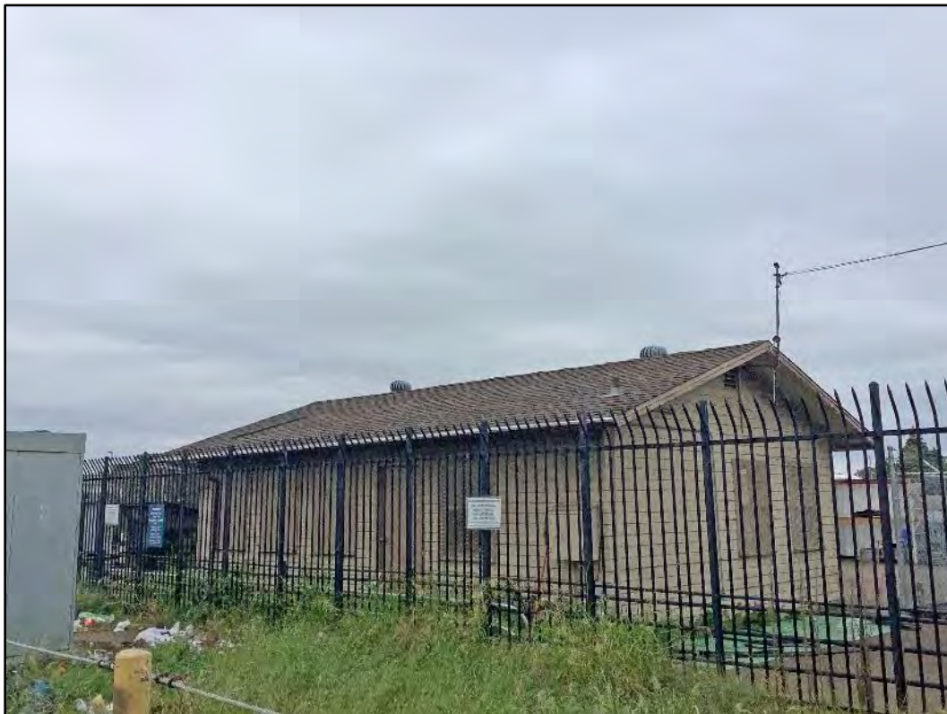
Figure 5.15-1 Building 34, Salvage Yard Office on Sports Arena Boulevard. Shows northwest and northeast façades, view toward the south.
