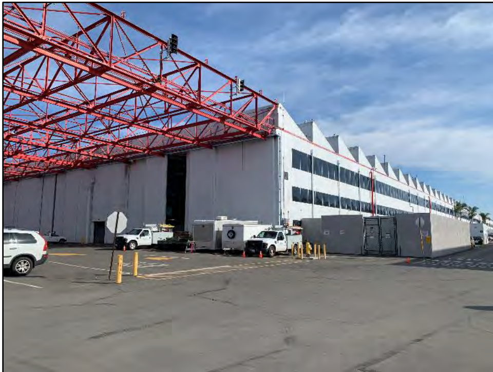
Image 1. Building 2, Exterior of the Northwest and Southwest Façades View toward the east.
