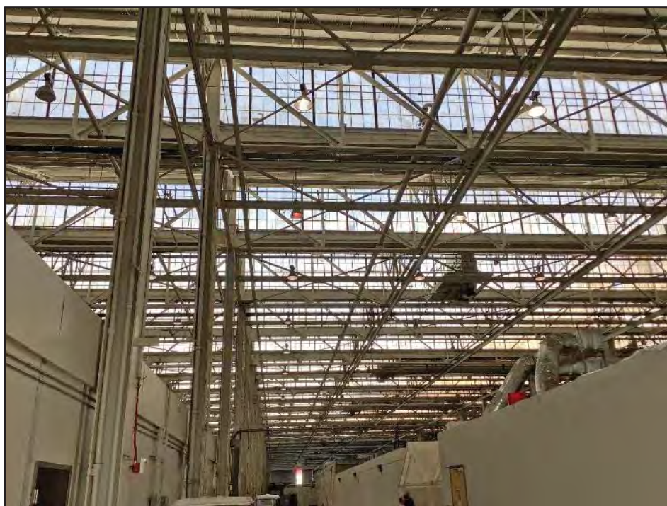
Image 3. Building 1 Interior, Showing Sawtooth Roof Window Arrangements and Suspended Lighting Fixtures. View toward the northwest.
