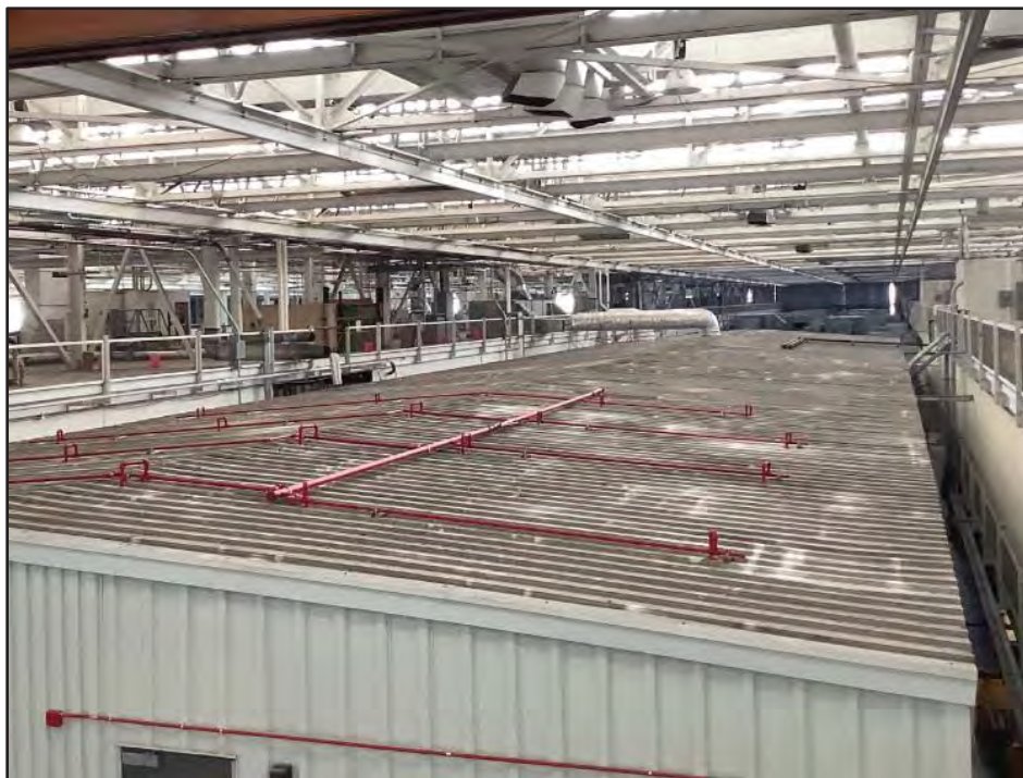
Image 8. Building 1 Interior, Corrugated Two-story Building Roof. Viewed from the third-floor mezzanine toward the northwest.
