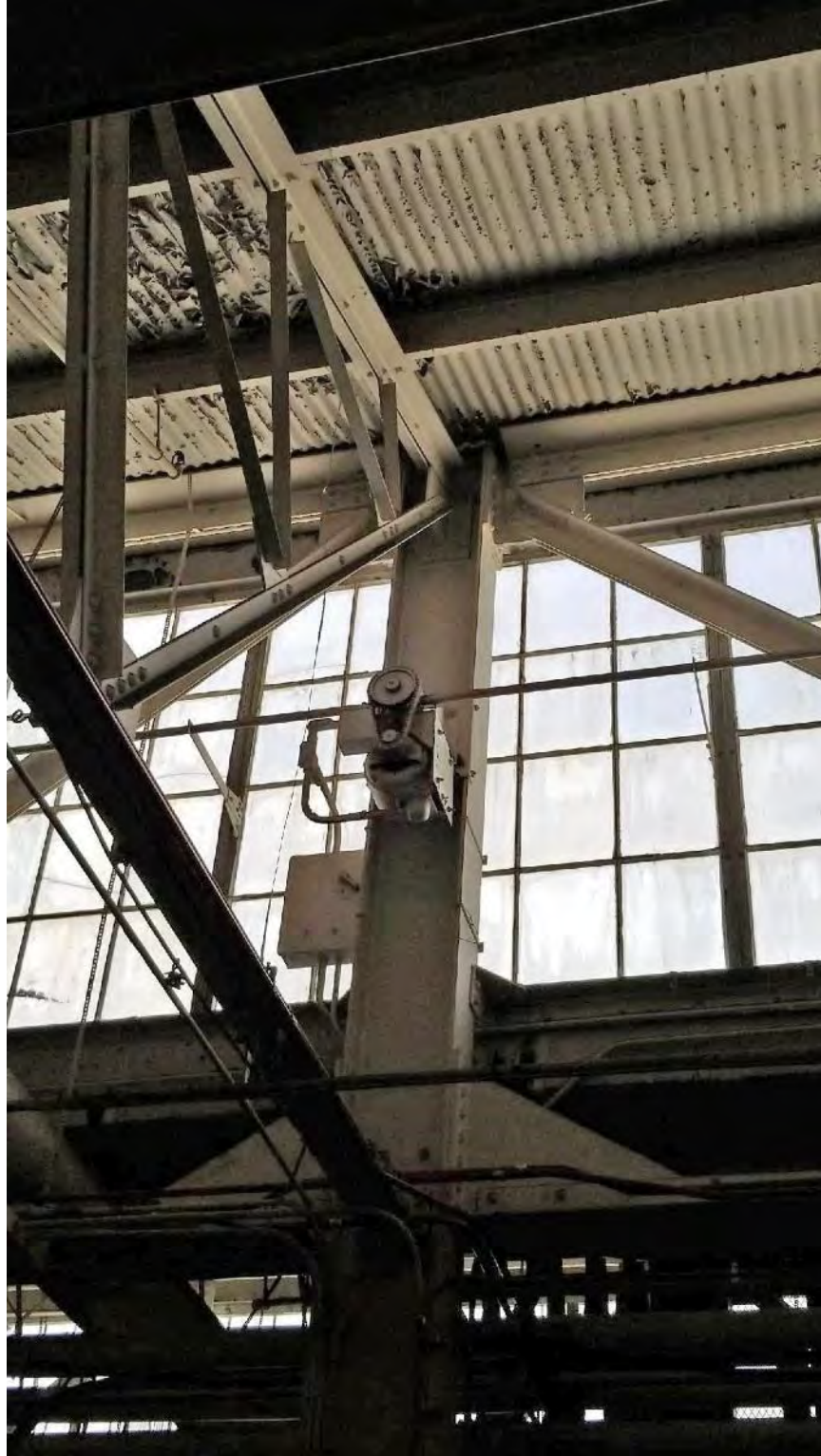
Figure 5.2-45 Building 3 Interior, Detail View of the Operating Mechanism of the Sawtooth Windows View toward the northwest.
