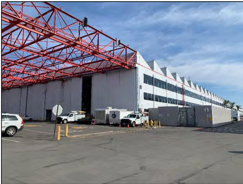
Figure 5.2-25 Building 2, Exterior of the Northwest and Southwest Façades View toward the east.
