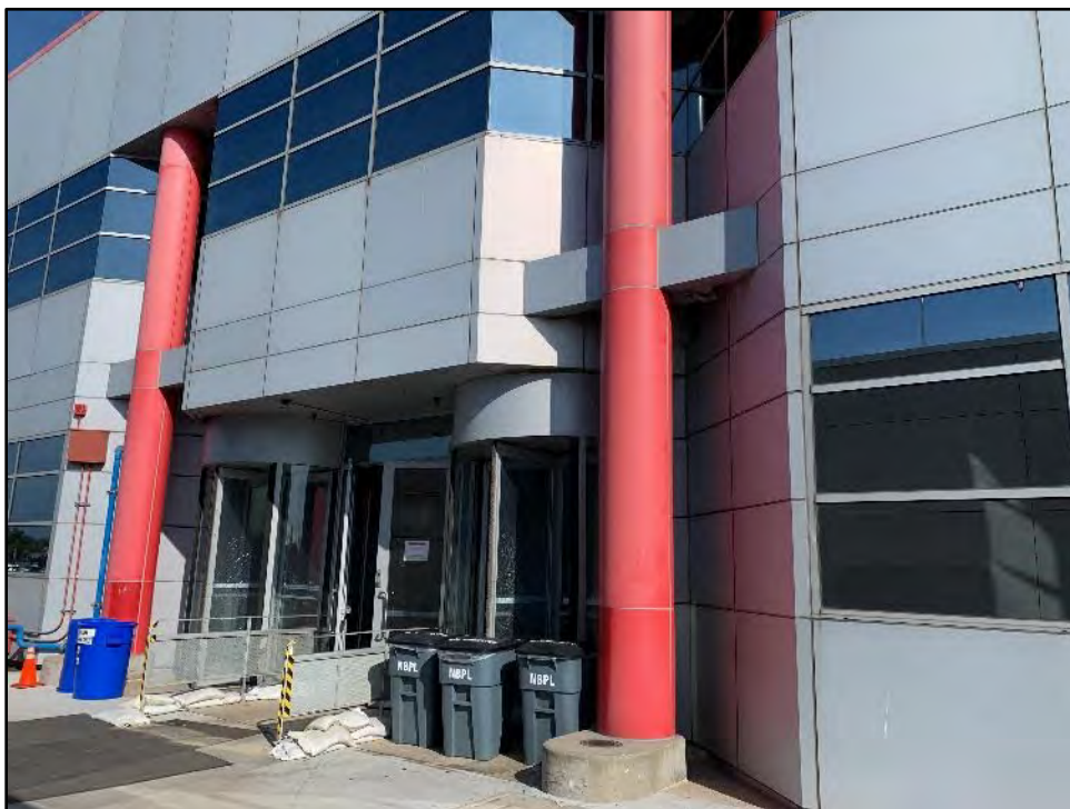
Figure 5.3-8 Building 4, Detail of Entrance at the Southwest Façade View toward the north.
