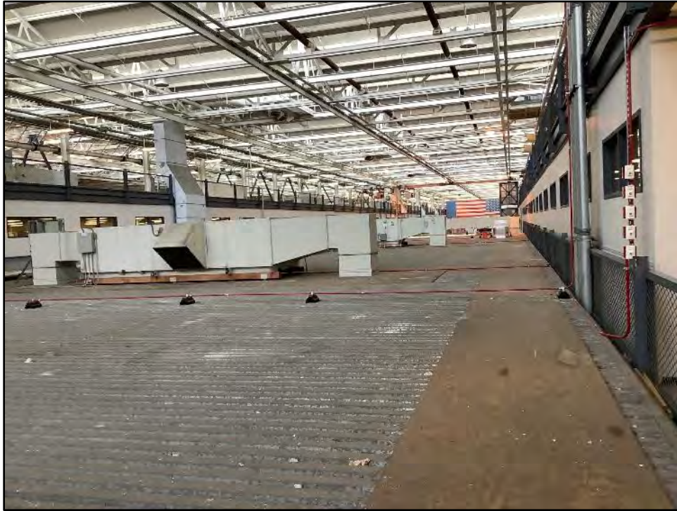
Figure 5.2-38 Building 2 Interior, Roof of Corrugated Building within the Main Building. View toward the southeast from the third floor mezzanine.
