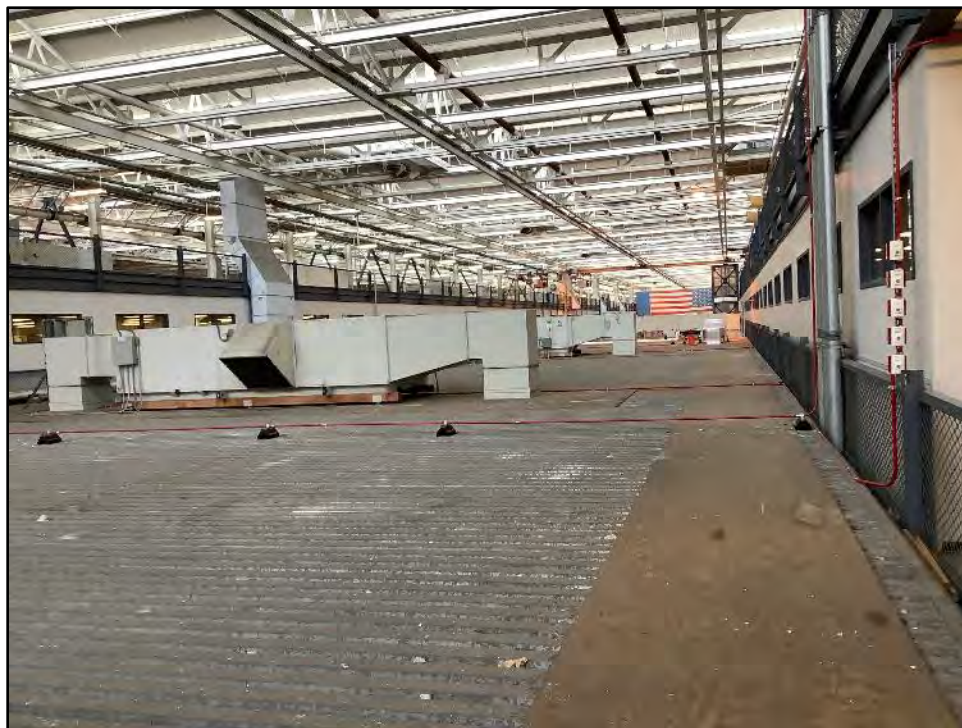
Image 6. Building 2 interior, roof of corrugated building within the main building. View toward the southeast from the third-floor mezzanine.
