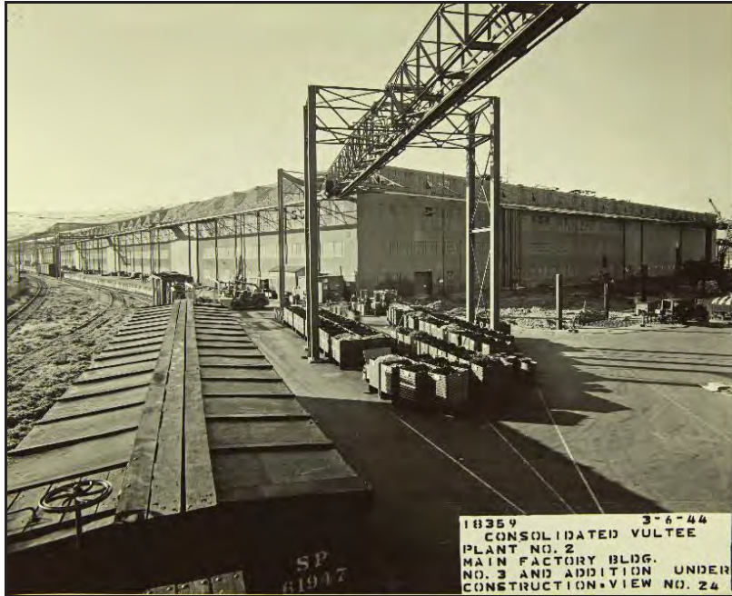
Image 1. Historical Photo of the Crane Monorail, showing trusses between buildings that ran along the northeastern façades of the manufacturing buildings, and also camouflage netting; view toward the south; March 6, 1944. Source: San Diego Air & Space Museum archives.
