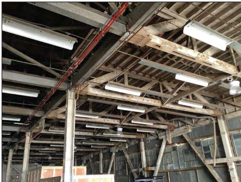
Image 8. Building 8 Interior, View from Roll-up Door at the Northwest Façade. View toward the southeast.
