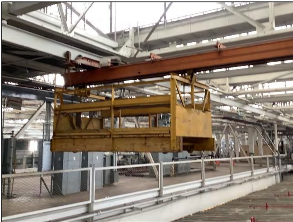
Figure 5.2-13 Building 1 Interior, with Detail of Underhung Crane and Suspended Hoist Mechanism View toward the northwest.
