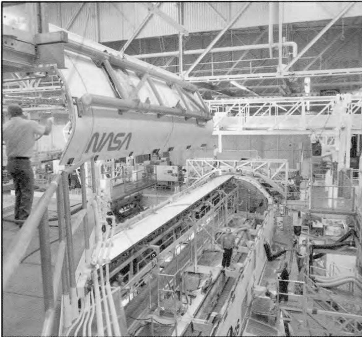
Figure 4.2-56 The Right Aft Payload Bay Door Segment being Lowered into Place on the Endeavor at Palmdale in the late 1990s
