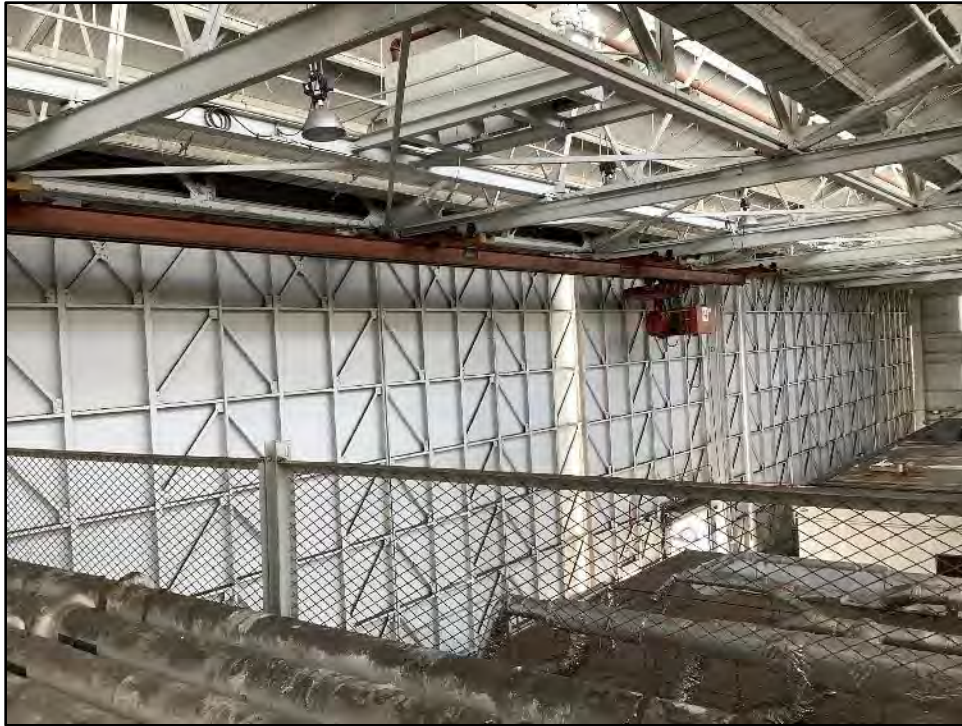
Figure 5.2-12 Building 1 Interior Showing Crew-operated Cab Suspended from Beam and Three-story Steel Hangar-type Doors Sliding View toward the south.
