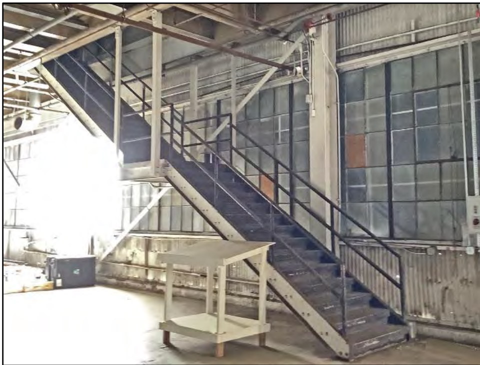
Figure 5.5-15 Building 8 Interior, Stairway from Ground Floor to Second Floor at Southwest Wall View toward the southeast.
