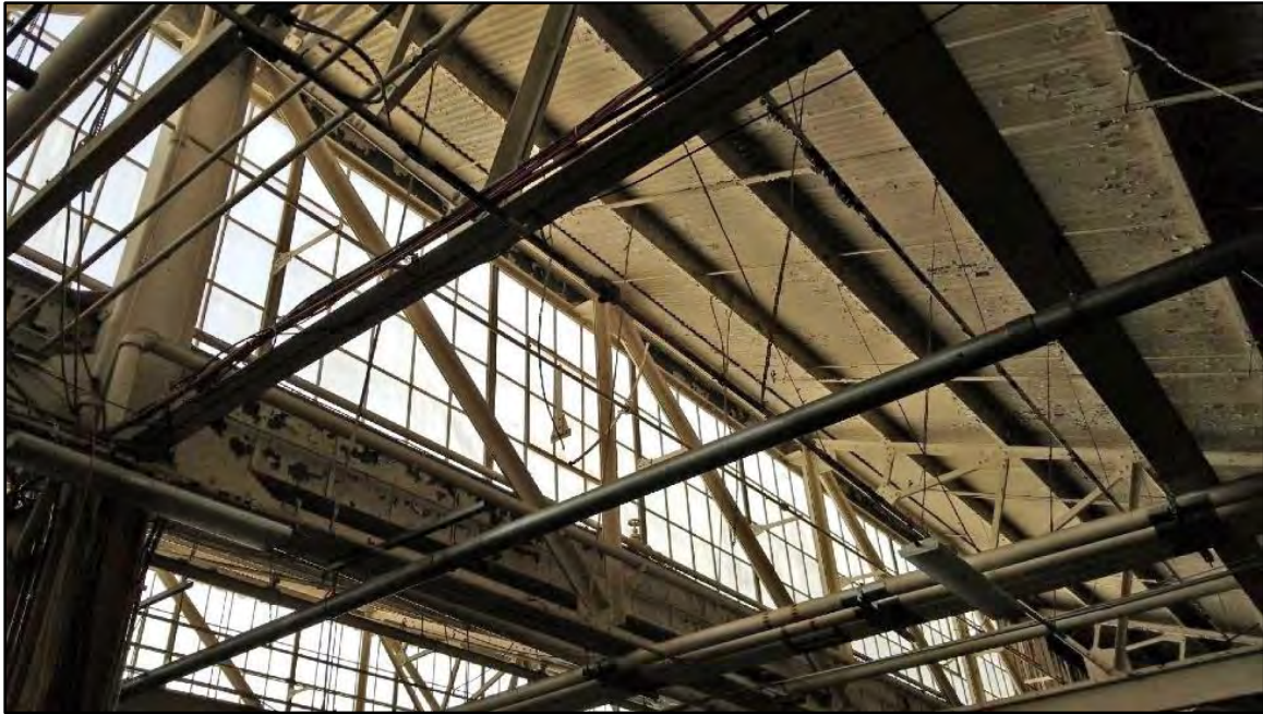
Image 4. Building 3 Interior, Showing Sawtooth Windows from the Highest Mezzanine. View toward the northeast.
