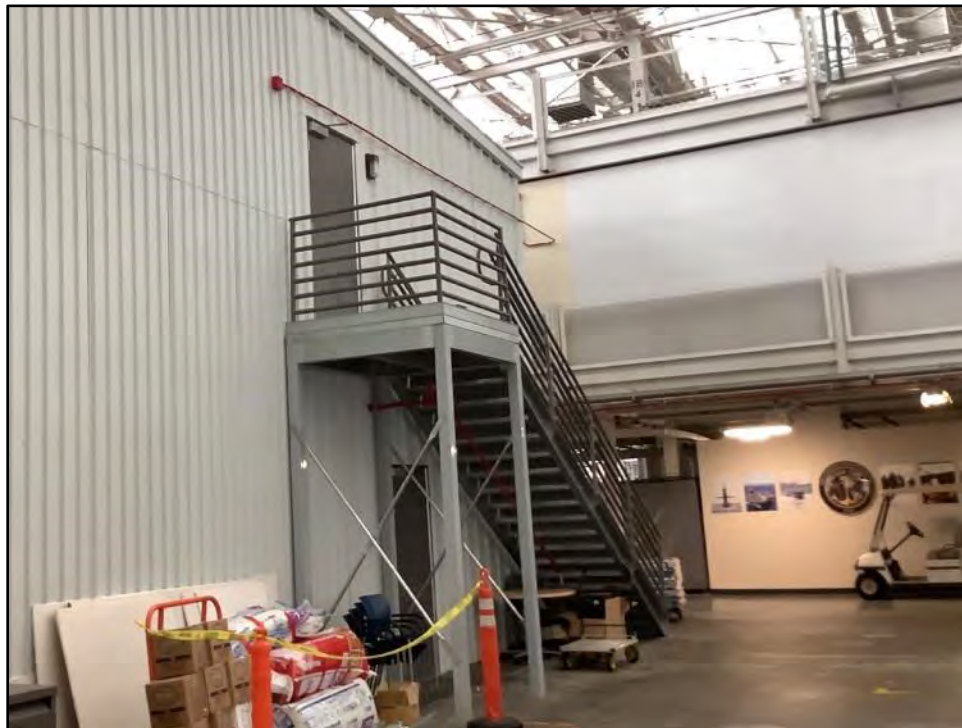
Figure 5.2-18 Building 1 Interior, Corrugated Two-story Building within the Main Building View toward the north.
