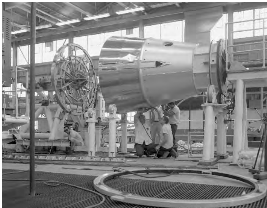
Figure 4.2-31 Cutting Skin, Building 3 (September 22, 1960) Courtesy of San Diego Air and Space Museum.
