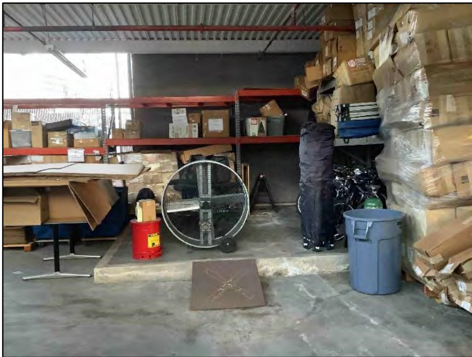
Figure 5.14-47 The Open Area at the North Façade of Building 4 Shows concrete slab for restroom, view toward the east.
