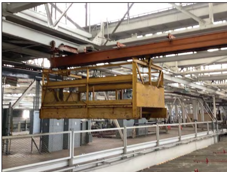
Image 5. Interior, with Detail of Underhung Crane and Suspended Hoist Mechanism. View toward the northwest.
