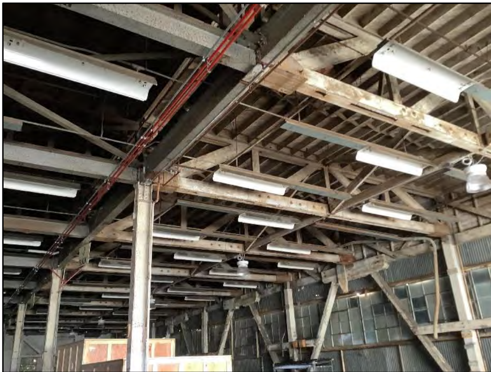
Figure 5.5-9 Building 8 Interior, View from Roll-up Door at the Northwest Façade View toward the southeast.
