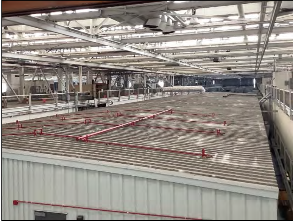
Figure 5.2-22 Building 1 Interior, Corrugated Two-story Building Roof Viewed from the third floor mezzanine toward the northwest.
