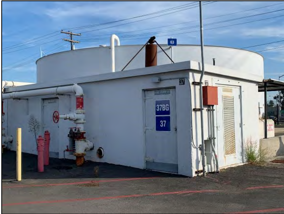
Figure 5.10-2 Detail of Building 37, the North and West Façades View toward the southeast.
