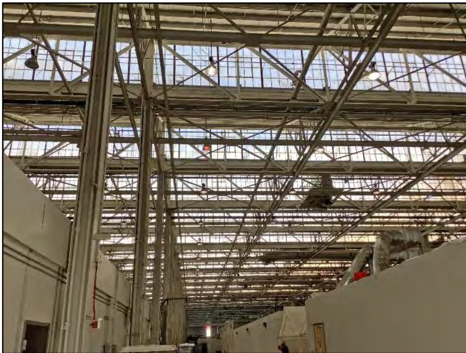
Figure 5.2-9 Building 1 Interior, Showing Sawtooth Roof Window Arrangements and Suspended Lighting Fixtures View toward the northwest.
