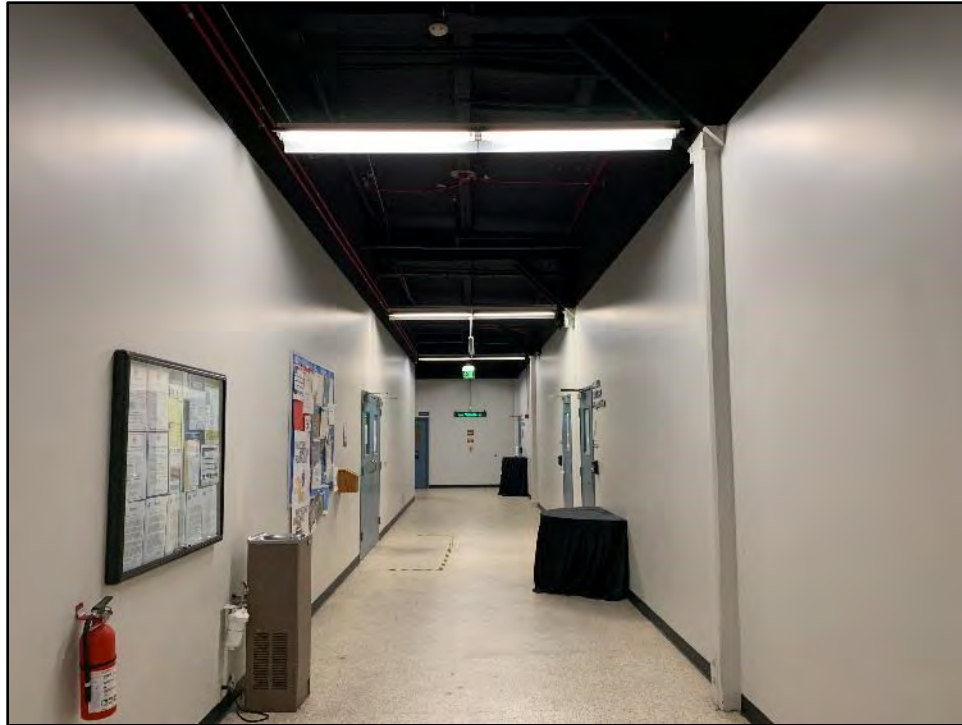
Figure 5.6-5 Building 27 Interior, Central Corridor at Northwest End of Building View toward the southeast.
